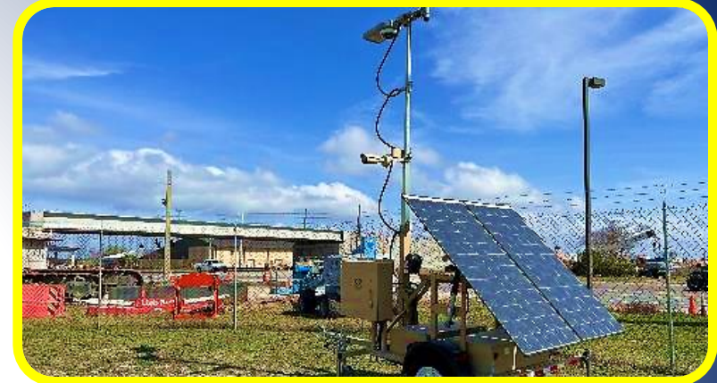
Valitus Modular LED streetlight with five 4K cameras originally purchased to detect unauthorized flight line access
